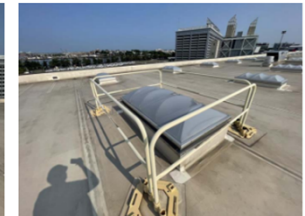
PHOTO 3: SMOKE HATCH ON ROOF AREA A.
