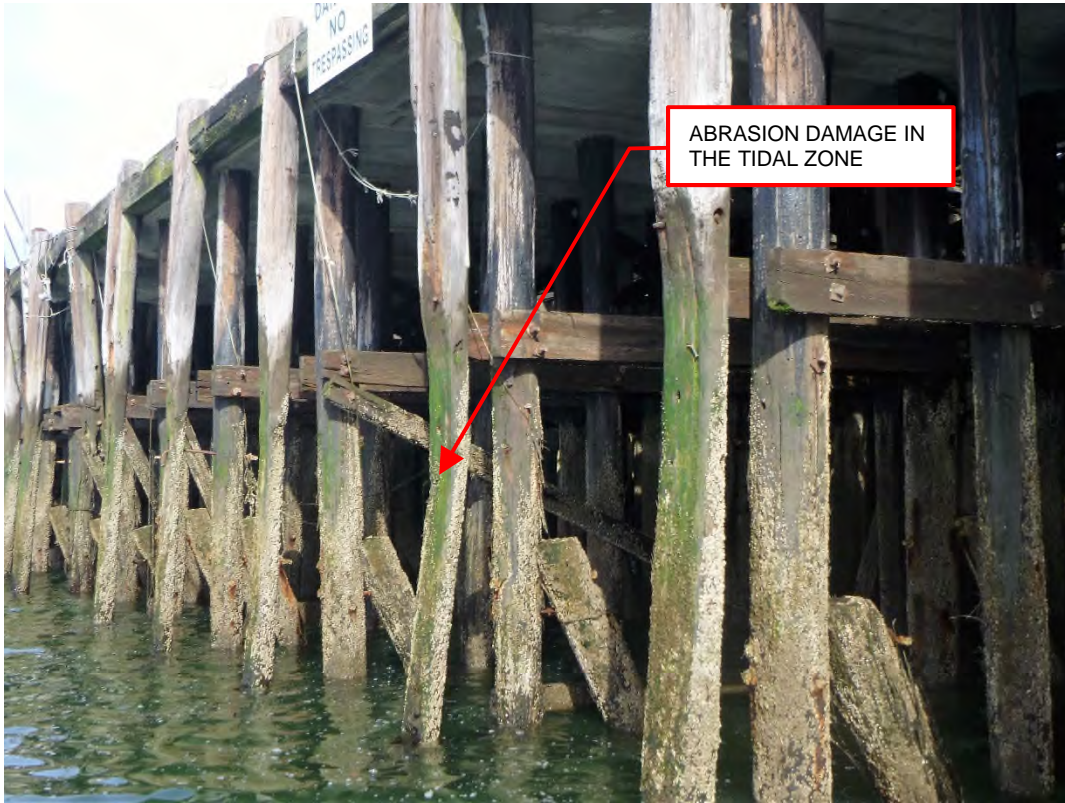
Photo 19 – Timber fender pile along the northwest berth of the pier.
