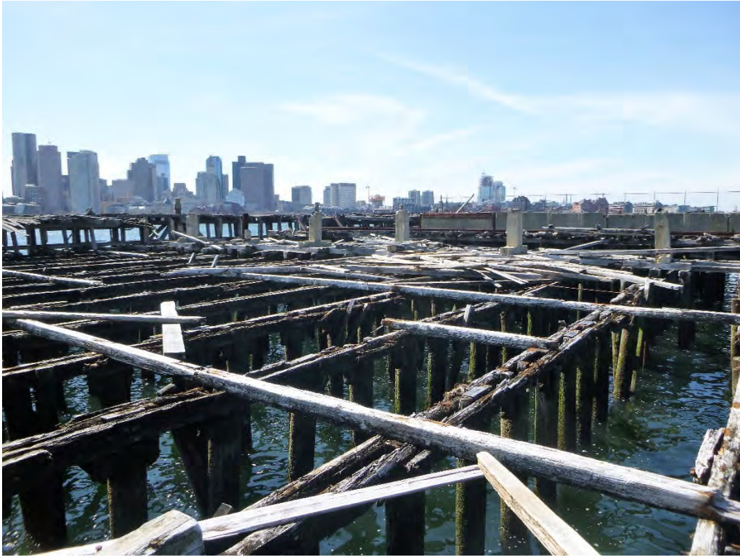
Photo 3 – Overall of missing decking to the outshore portion of the pier.
