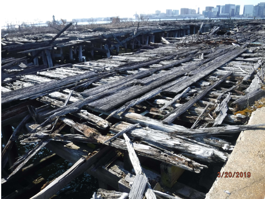
Photograph 3: View of the western side of Pier 3, facing south from the backlands.
