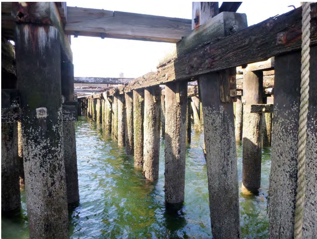
Photo 16 – Overall condition of timber piles along a typical bent outshore of the pier.
