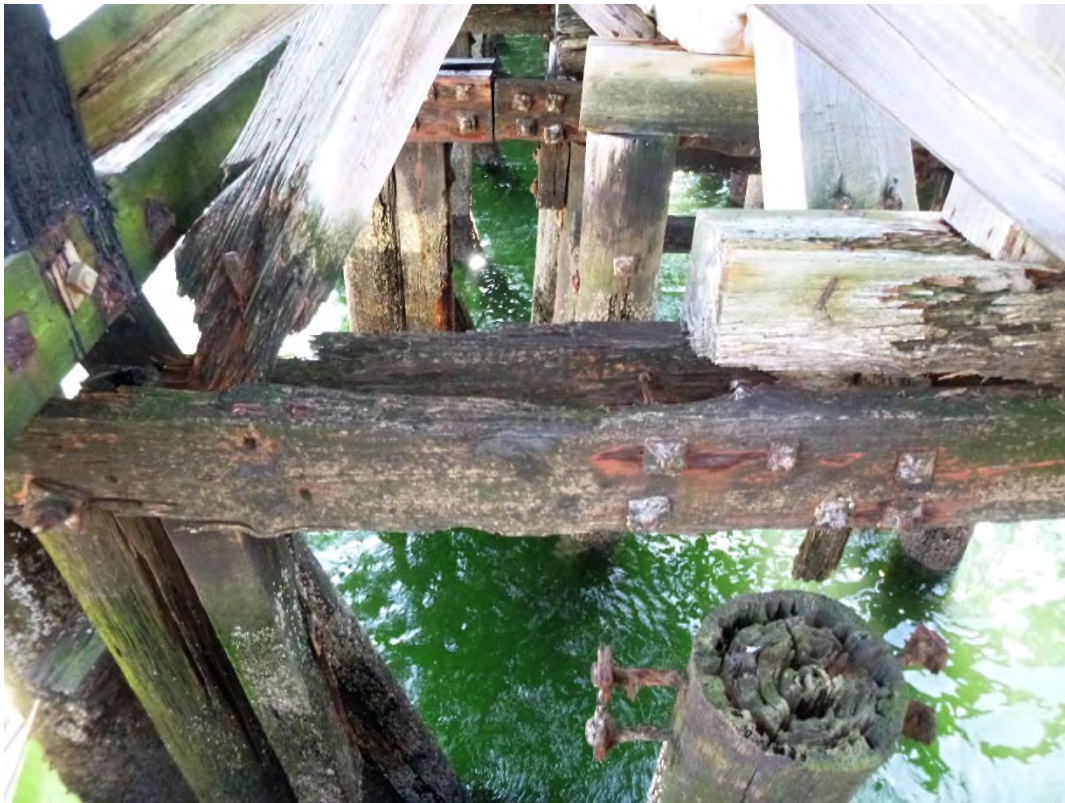
Photo 8 – Deteriorated sections of timber pile cap and adjoining timber bracing under deck apron, on the southeast side of the pier.
