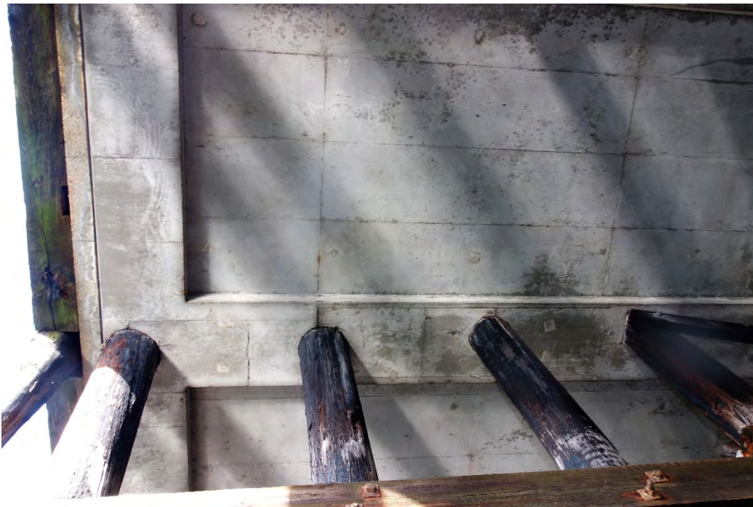
Photo 2 – Typical condition of the concrete apron deck on the northwest side of the pier.
