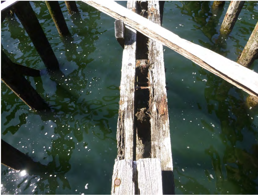
Photo 9 – Typical condition of interior timber pile cap with fungal decay.
