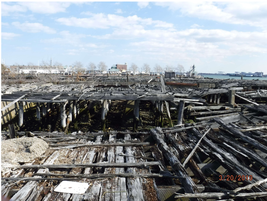
Photograph 4: View of the center of Pier 3, facing east from the western apron.
