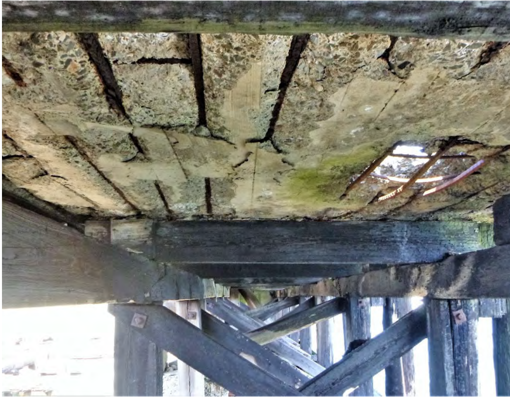
Photo 1 – Open corrosion spalling under concrete apron deck on the southeast side of the pier.
