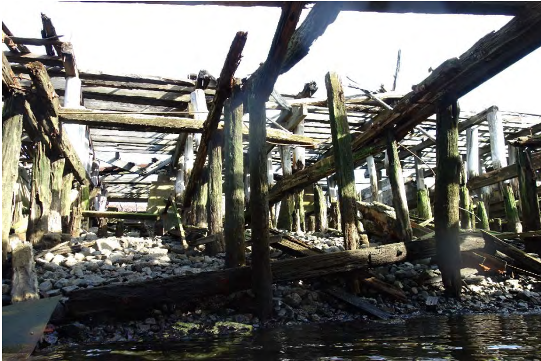
Photo 20 – Earth core on the northwest side of the pier, with debris and structural remnants.
