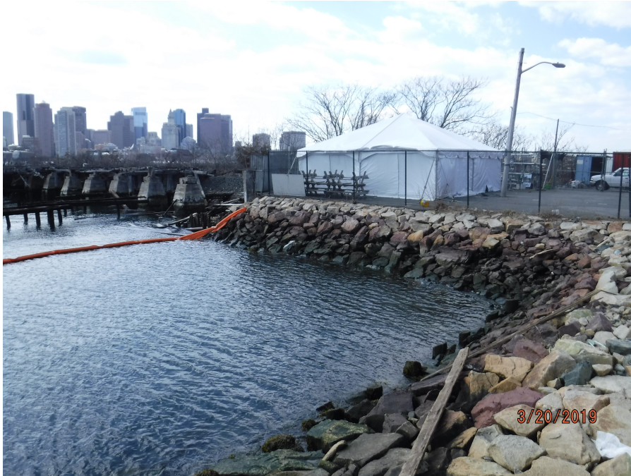
Photograph 9: View of stone riprap along the intertidal zone, south of Sailing Center, facing west.
