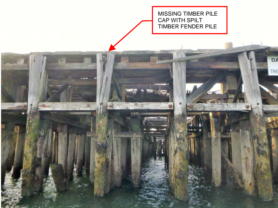
Photo 18 – Typical condition of timber fender system along the southeast berth of the pier.
