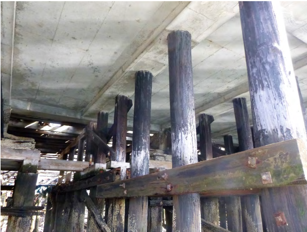
Photo 14 – Typical timber piles beneath the concrete apron of the northwest side of the pier, looking South.
