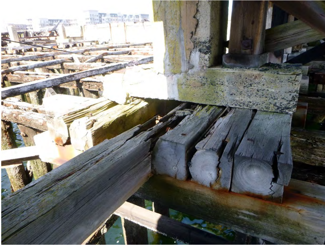
Photo 7 – Typical condition of timber cribbing beneath concrete pedestal with fungal decay.
