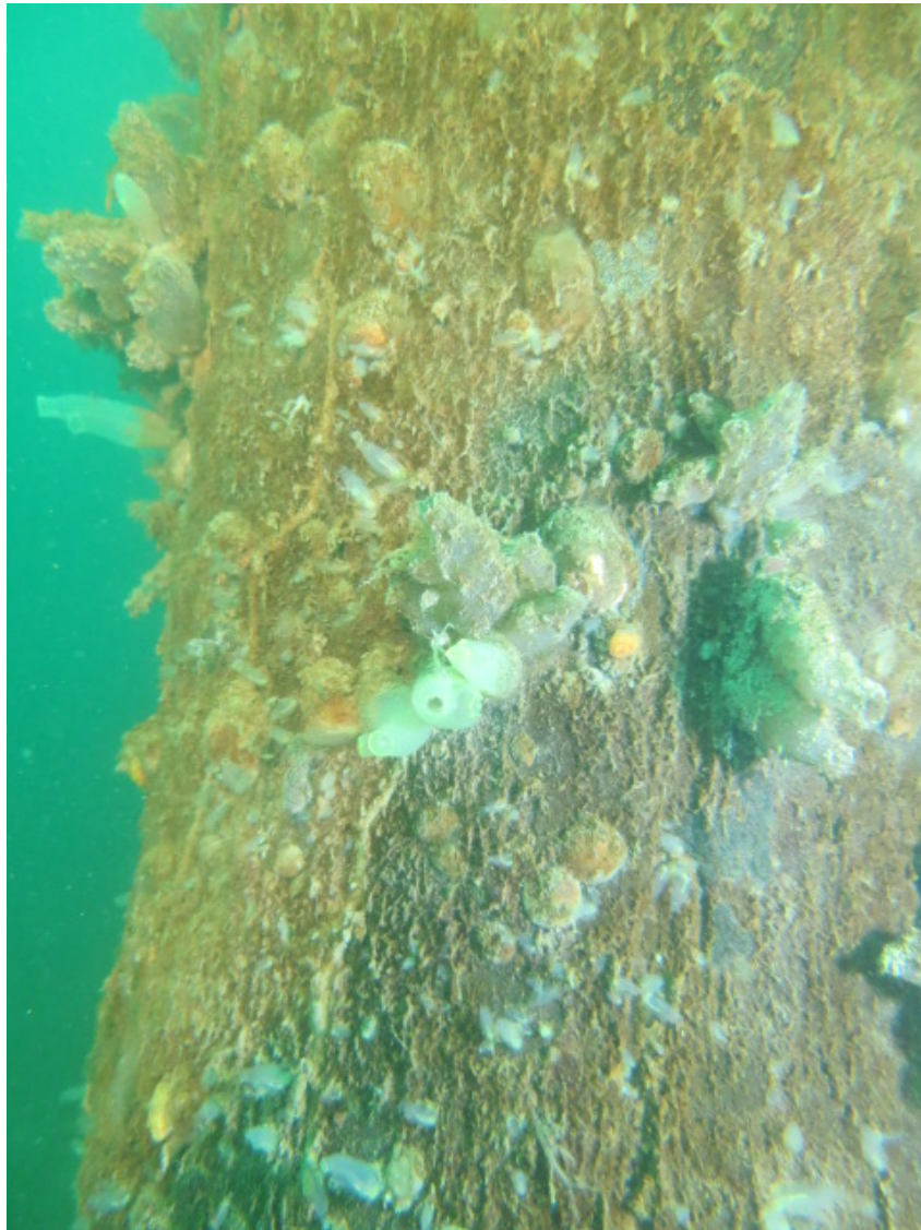
Photograph 17: Typical view of sponges and tunicates on piers/piles along Pier 3.
