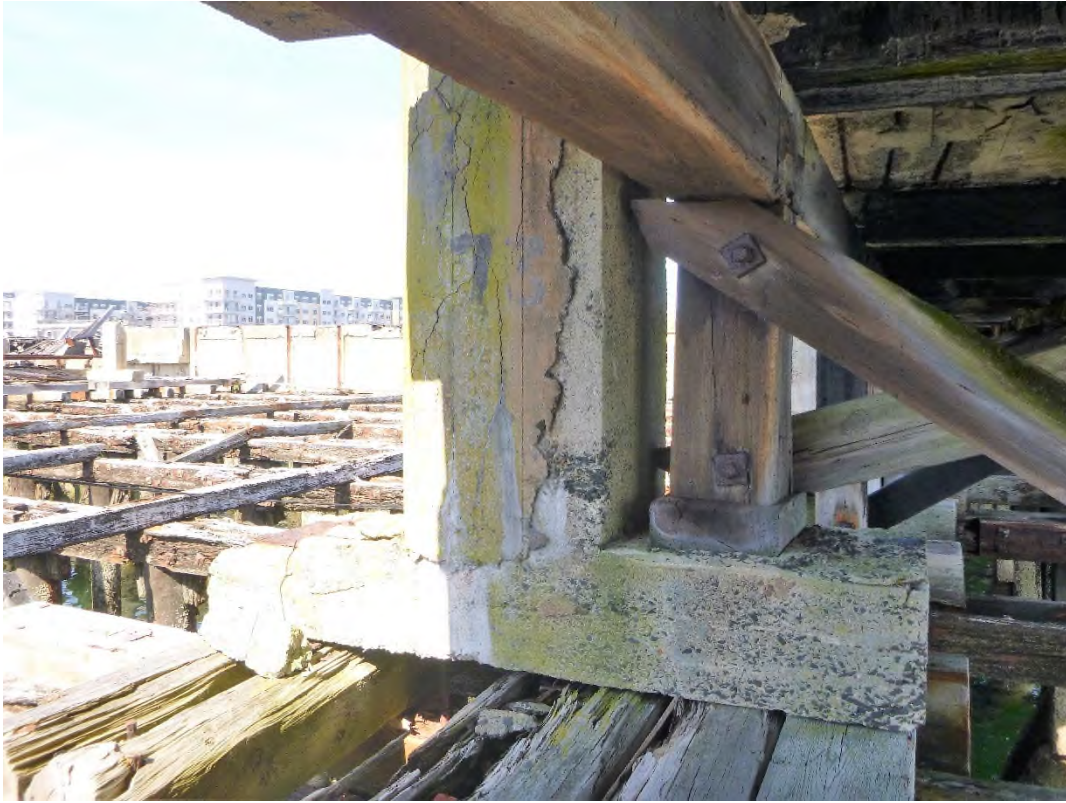
Photo 5 – Typical concrete pedestal under deck apron on the southeast side of the pier.
