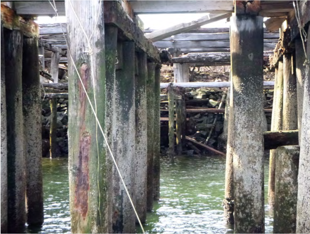
Photo 13 – Typical timber piles beneath the concrete apron of the southeast side of the pier.
