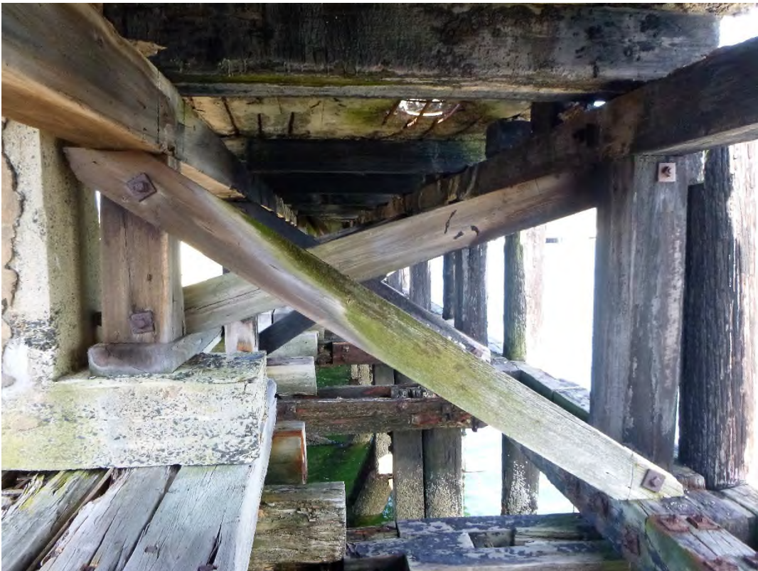
Photo 6 – Timber sub structure framing under deck apron on the southeast side of the pier.
