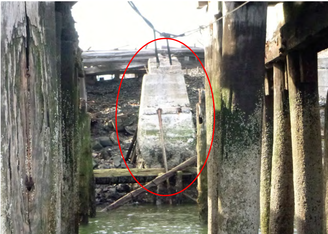
Photo 4 – Typical large interior concrete pedestal near the inshore portion of the pier.
