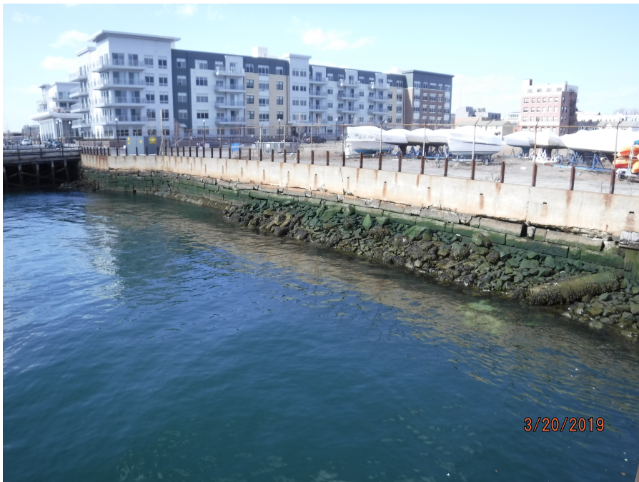
Photograph 10: View of stone riprap along the intertidal zone and seawalls, along western limit of Study Area, facing north.
