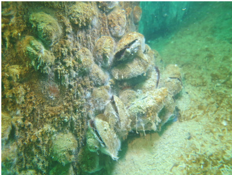
Photograph 12 : Typical view of shellfish (blue mussels) at base of piers/piles along Pier 3.
