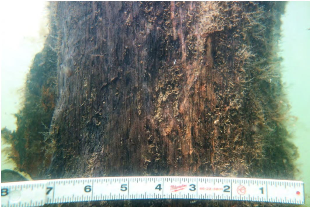
Photo 12 – Typical condition of interior pile below water with marine borer damage.
