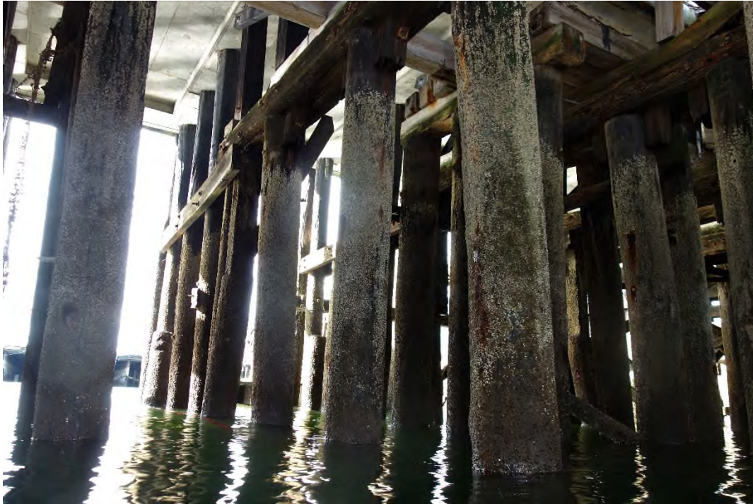
Photo 15 – Typical timber piles beneath the concrete apron of the northwest side of the pier, looking North.
