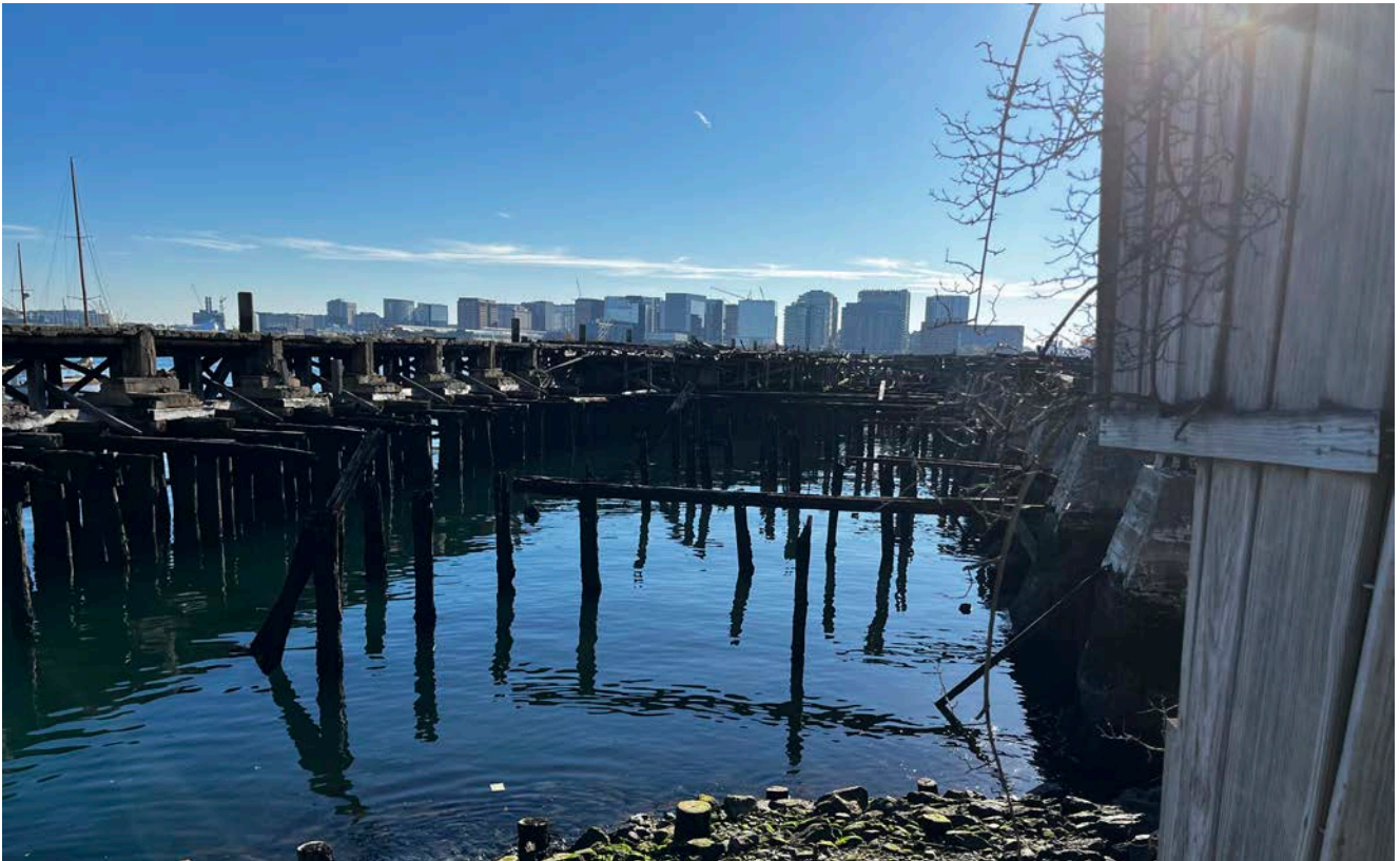
Photograph 1: Looking southwest from the Sailing Center's rental tent towards the Project Site.
