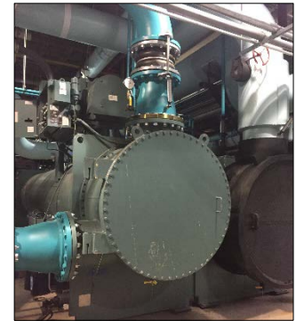
New Chiller at Central Heating and Cooling Plant
