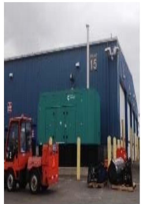
Emergency Diesel Generator at Building 15, Logan Airport
