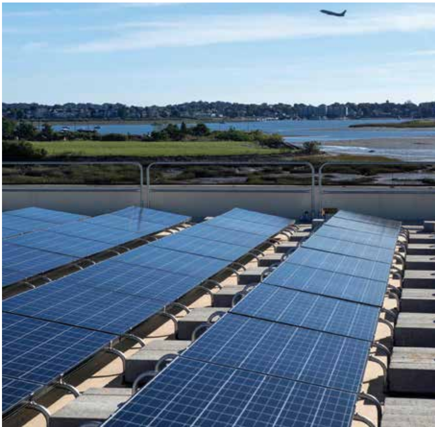
Solar panels at the Green Bus Depot.
