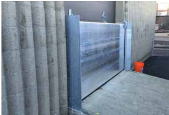
Flood barriers help protect from storm surge at Boston Logan International Airport
