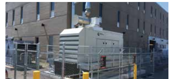
Electrical generators are elevated above flood levels at the State Police headquarters
