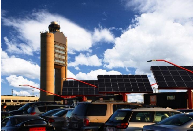
Solar Panels on the roof of Terminal B Garage. Source: Massport.
